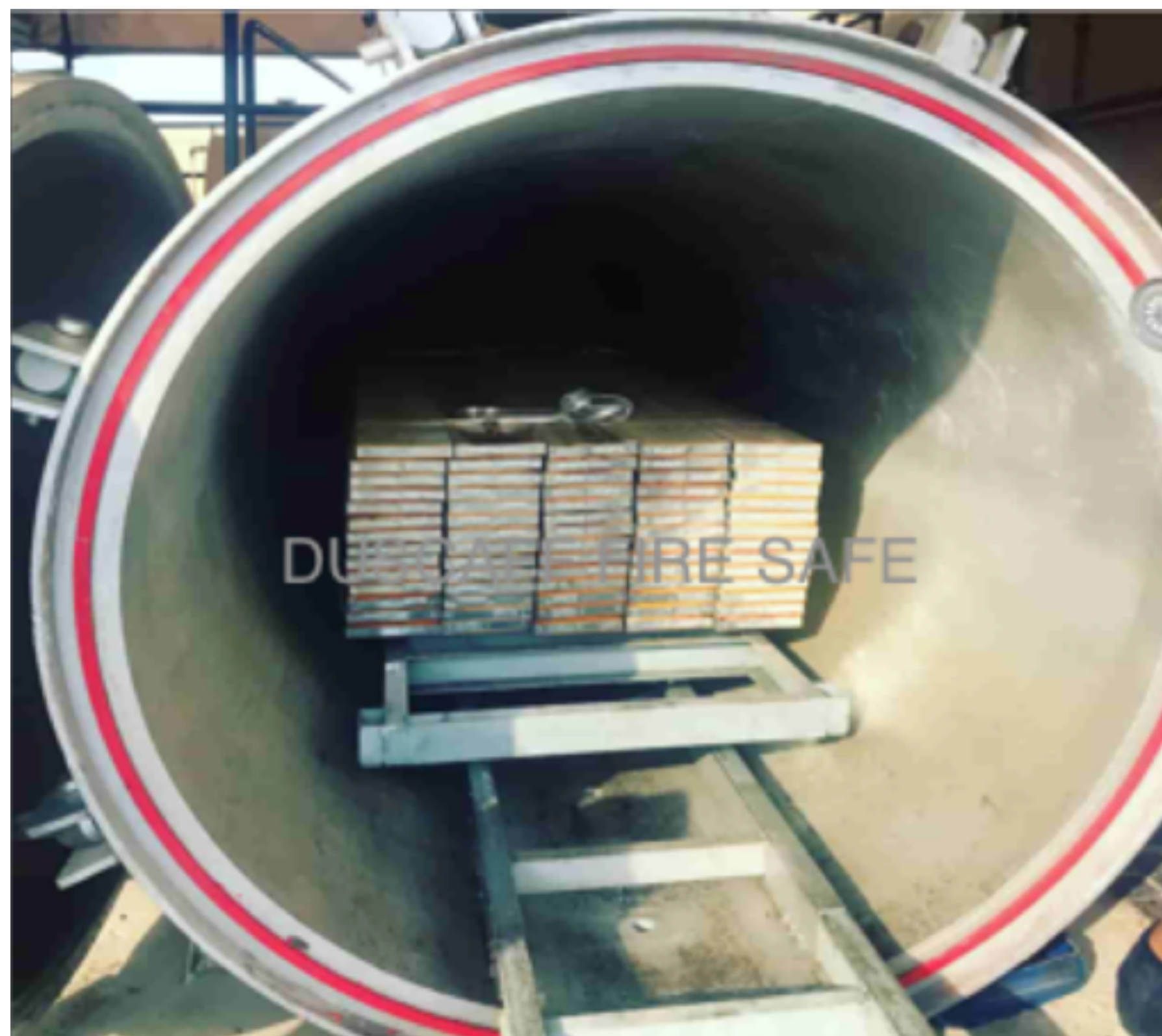
SW Range in the pressure treatment plant
